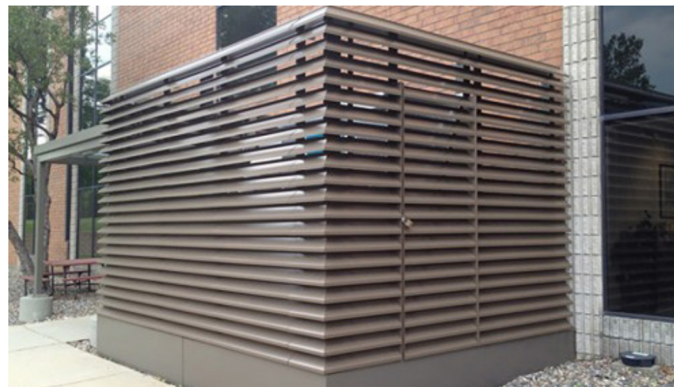
FIGURE 1.12 EQUIPMENT AND TRASH SCREENING EXAMPLES
