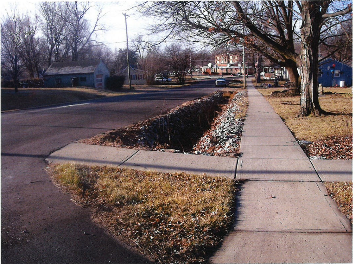
Photo 31 - Image open storm water drainage ditch. Note no railings or bollards preventing vehicular or pedestrian access/accidents. Also note lack of truncated pedestrian strip at sidewalk crossing.
