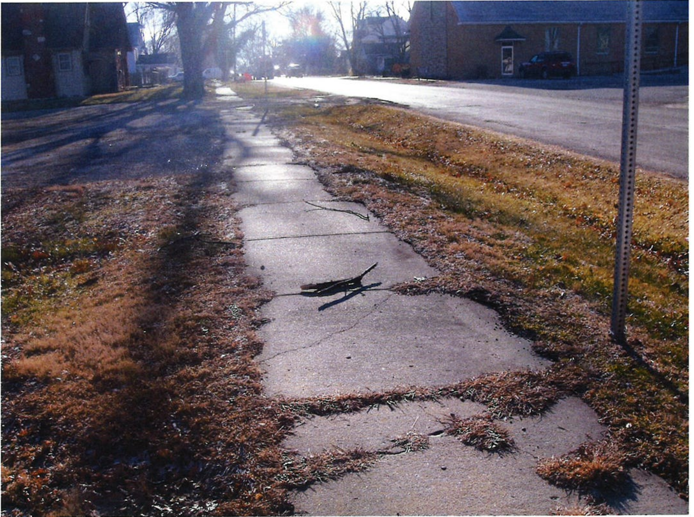
Photo 37 - Typical view of sidewalk condition within the Redevelopment Area.
