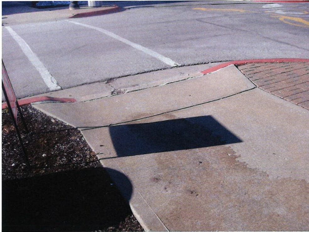
Photo 3 - Main Street pedestrian crossing ramp. Note lack of detectable truncated dome warning strips for visually impaired individuals.
