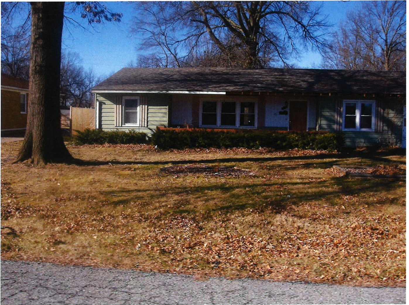
Photo 51 - Deteriorated single-family residence. Note missing roof soffit. Also, damaged downspout to left of structure. Continued neglect of this issue could lead to inadequate water drainage from structure, possibly compromising the integrity of the residence.
