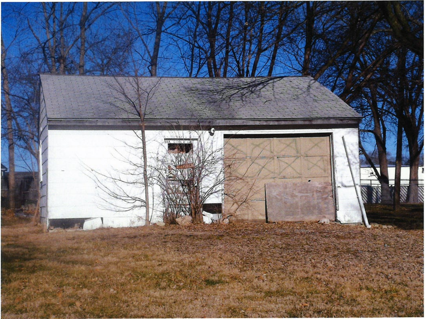
Photo 42 - Deteriorated/damaged garage structure. Also note lack of vehicle drive to structure. Condition is an indication of lack of regular property maintenance. This condition may lead to an economic and social liability and may be conducive to the ability to pay reasonable taxes.
