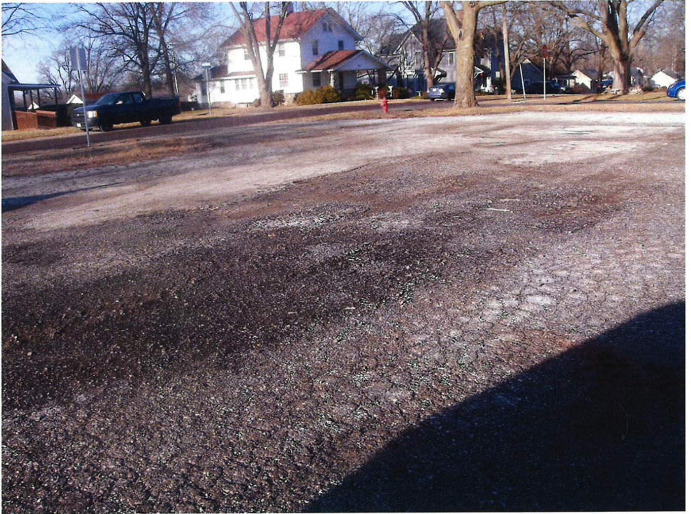
Photo 23 – Image showing deteriorated parking lot.
