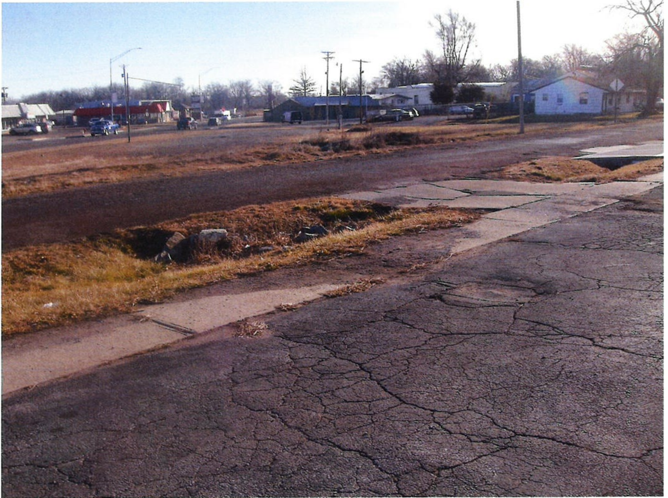
Photo 24 – Image showing deteriorated public and private infrastructure. Note deteriorated nature of sidewalk and drainage culvert. Also note deteriorated drive approach and surface parking.
