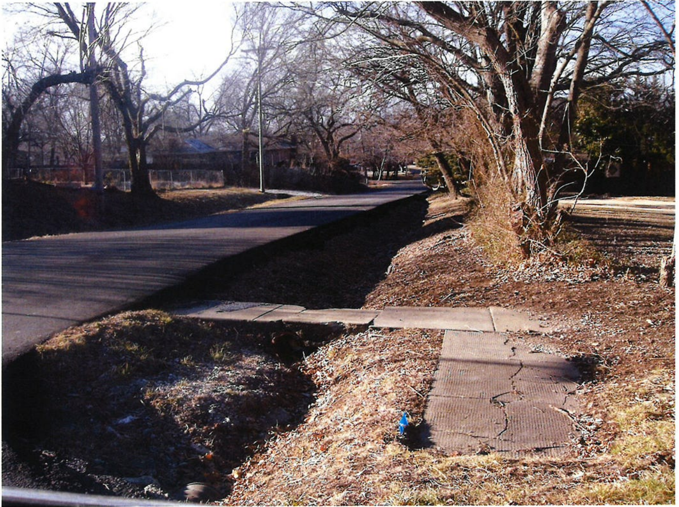
Photo 33 - Image open storm water drainage ditch. Note no bollards preventing vehicular accidents. Also note lack of pedestrian sidewalk continuation and deteriorated nature of sidewalk.
