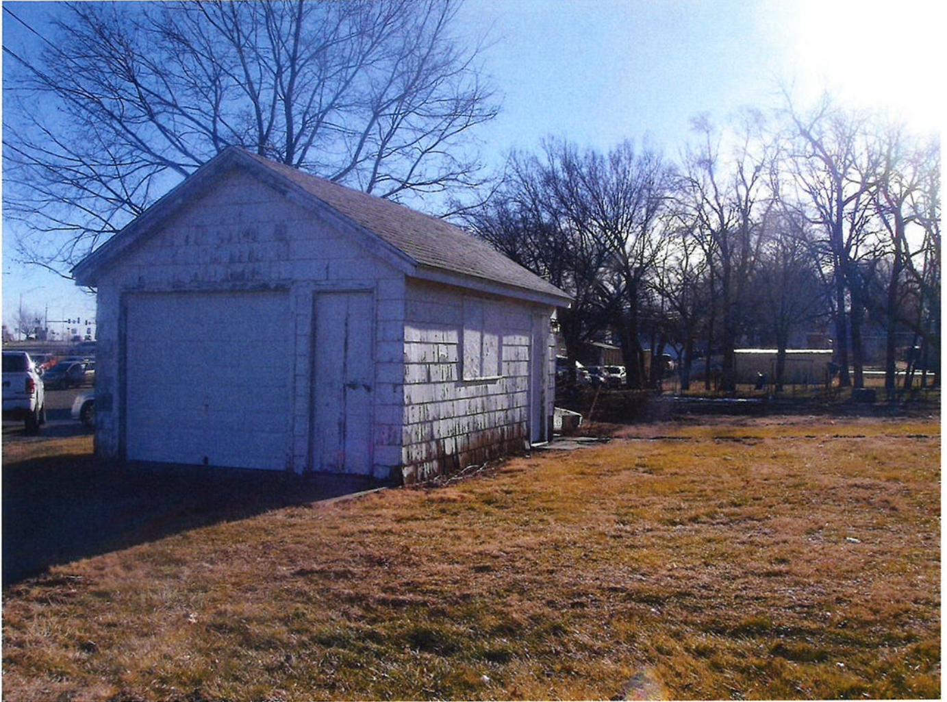
Photo 48 - Deteriorated garage structure. Condition is an indication of lack of regular property maintenance. This condition may lead to an economic and social liability and may be conducive to the ability to pay reasonable taxes.
