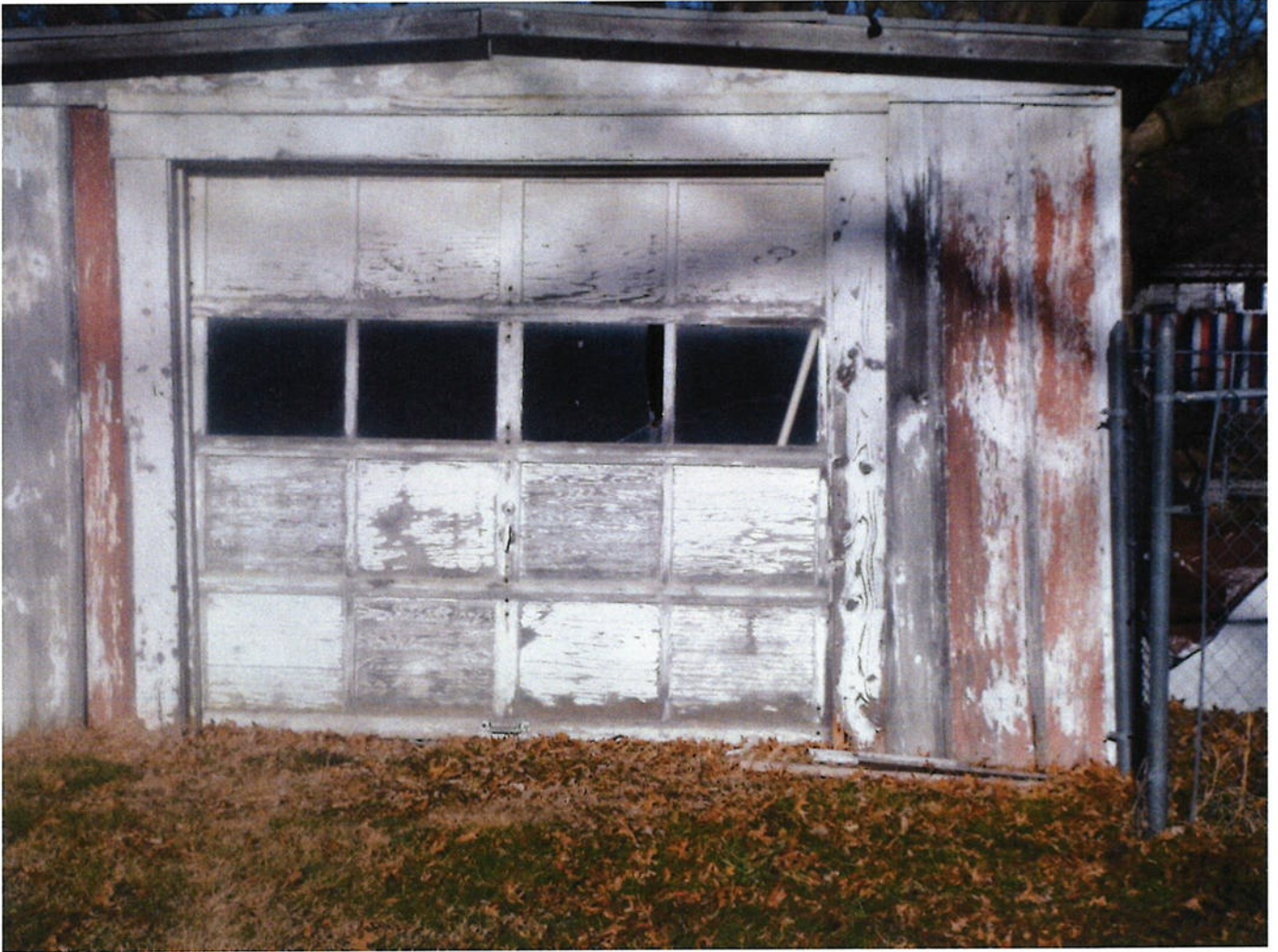
Photo 43 - Deteriorated/damaged garage structure. Also note lack of vehicle drive to structure.
