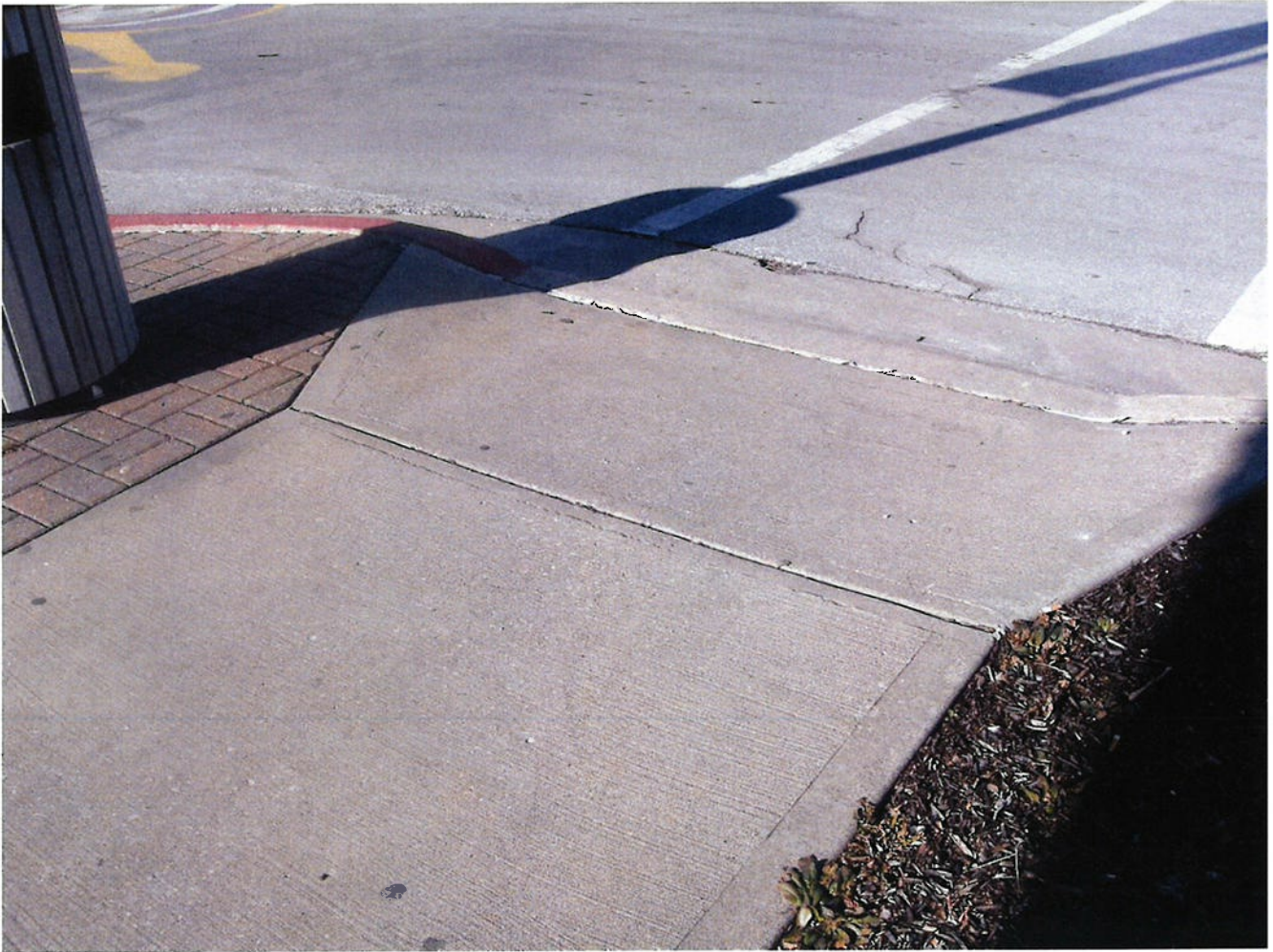
Photo 26 – Image showing pedestrian ramp with no truncated rumble strip.
