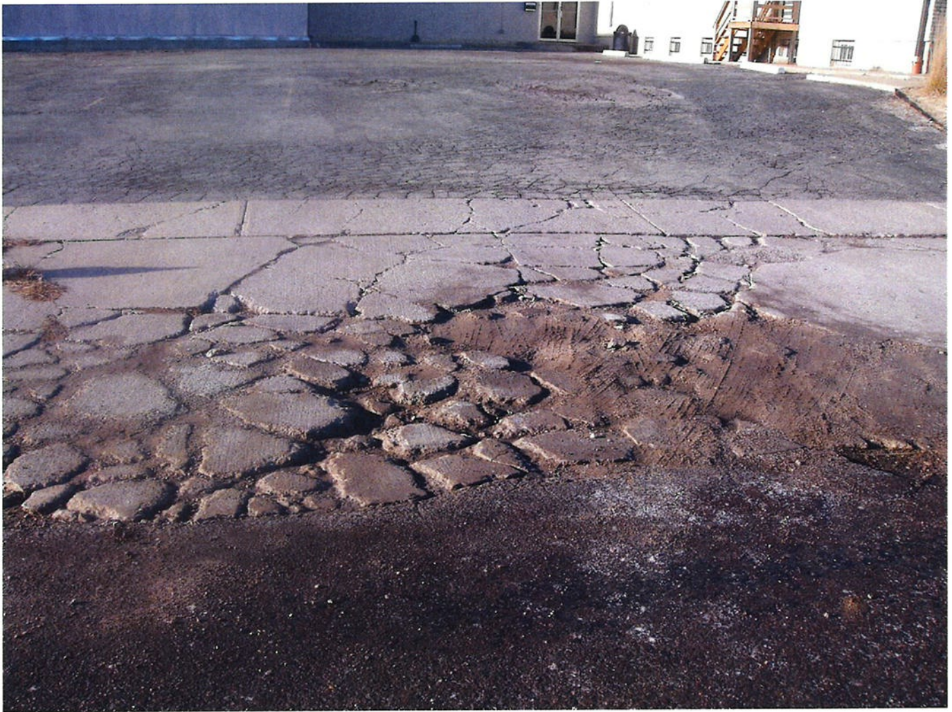
Photo 22 – Image showing deteriorated parking lot approach drive.
