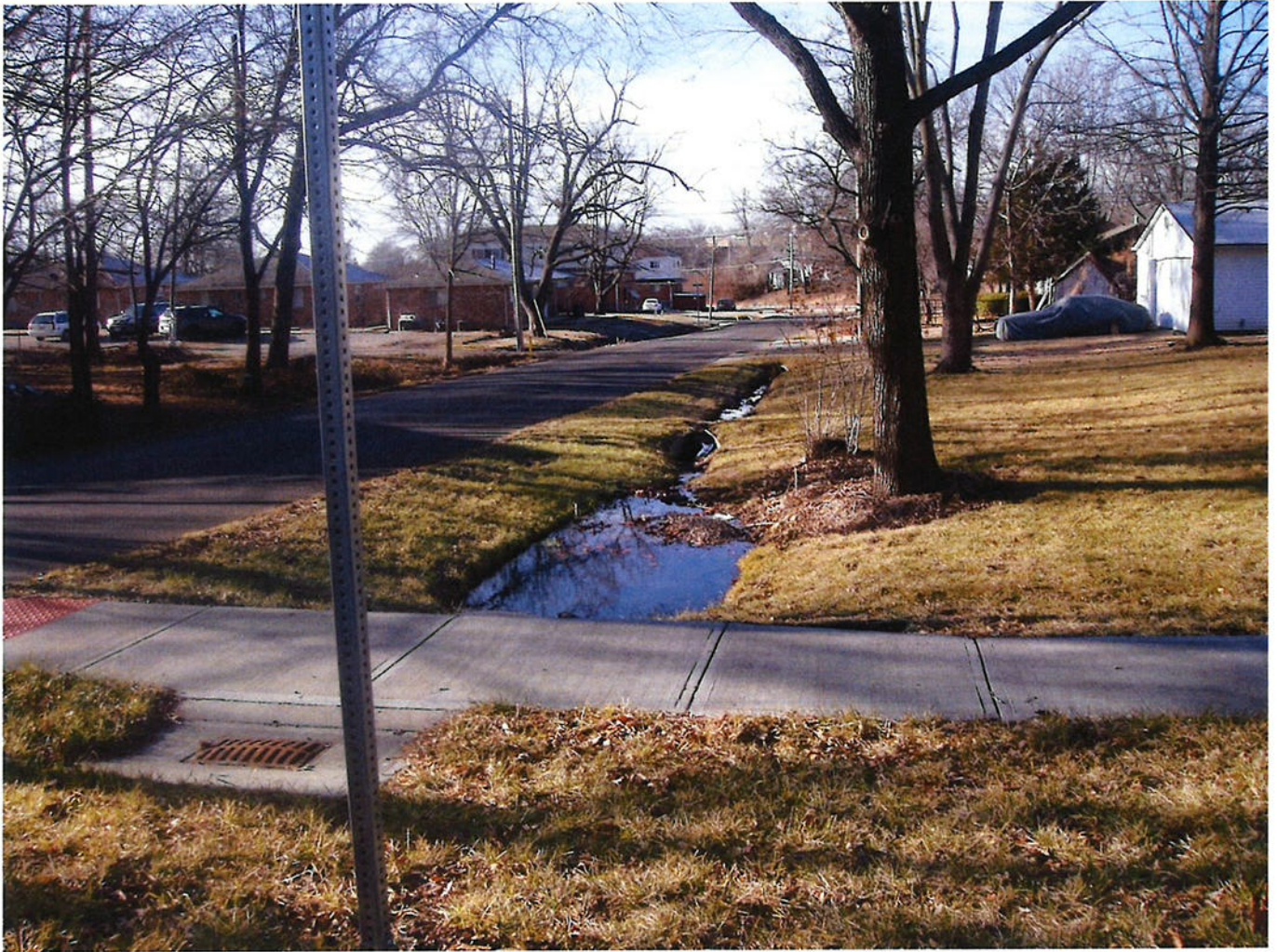
Photo 32 - Image open storm water drainage ditch. Note standing water, likely due to snow melt. Also note truncated pedestrian strip at sidewalk crossing.
