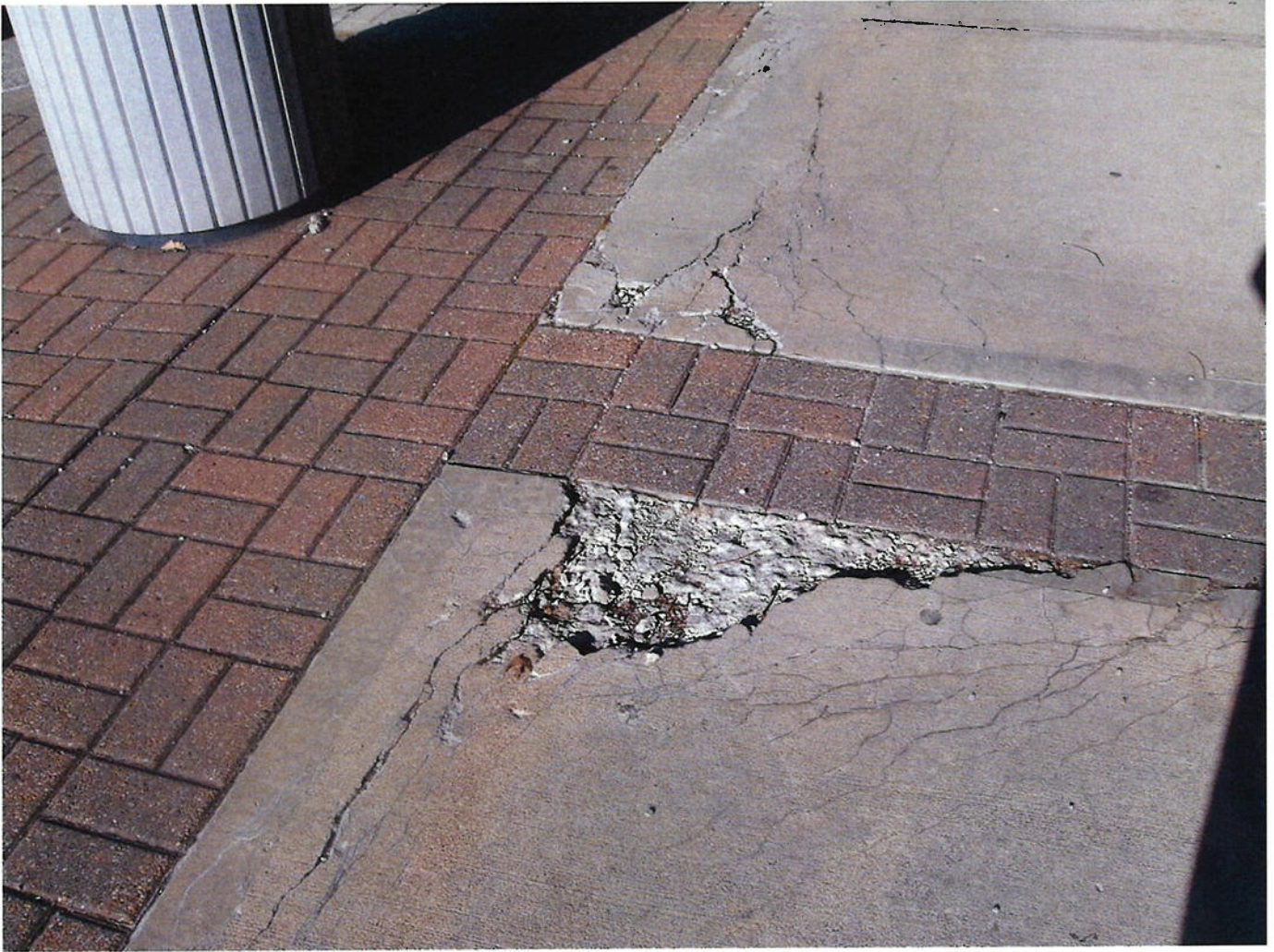
Photo 25 – Image showing damaged, deteriorated sidewalk.
