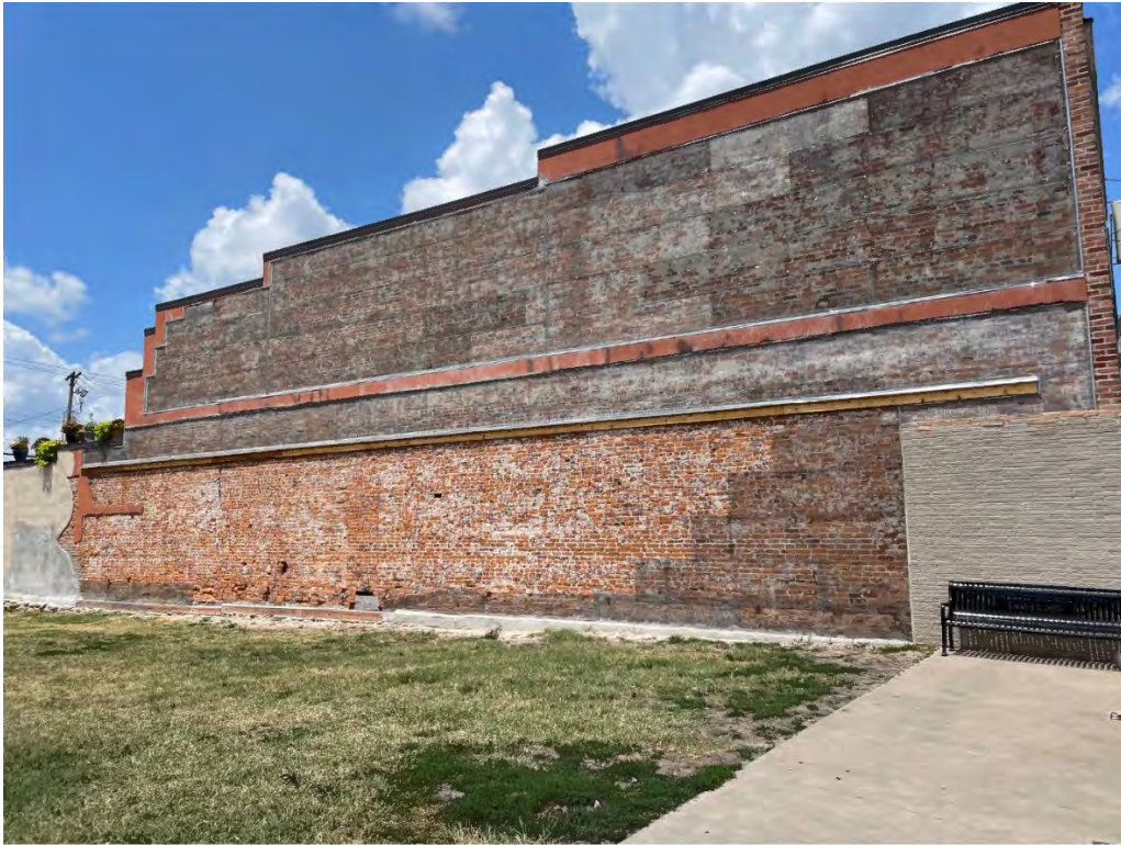
Side wall photo (stucco proposed on upper 15'; tuckpoint/repair of original brick on lower 13')
