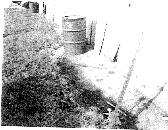
Photo #49 55-gallon drum containing water and staining at the edge of the concrete
