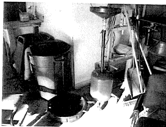
Photo #76 Used oil collection system
