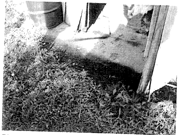
Photo #50 Staining at the edge of the concrete
